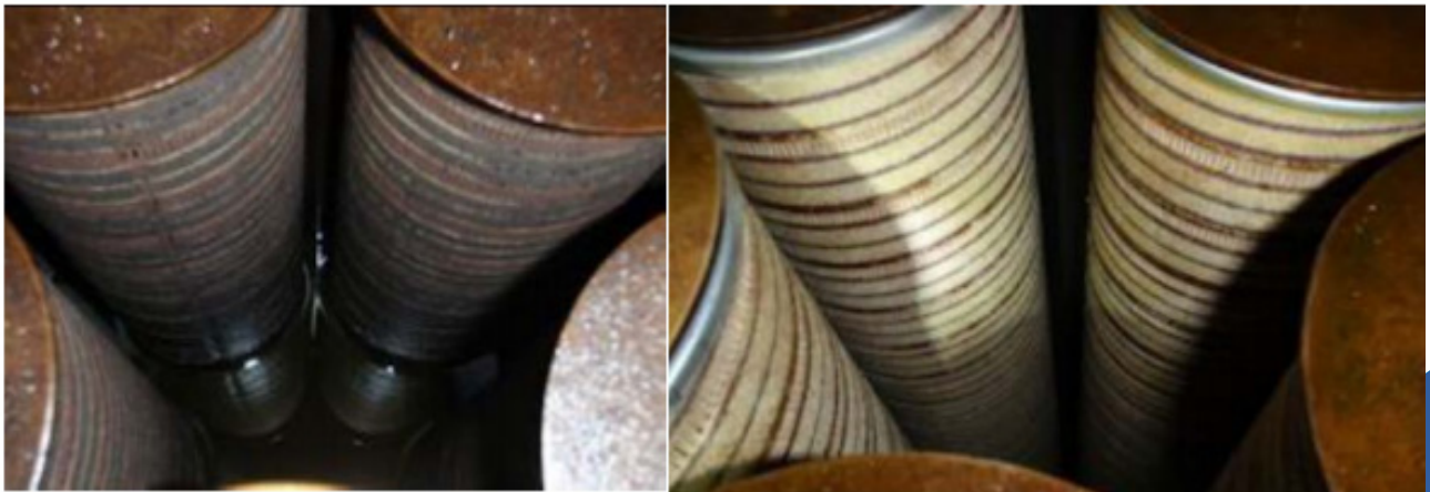
The filters were significantly cleaned along with the other system components during the flush
